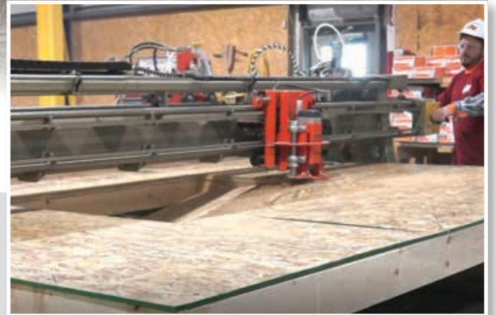
Automated routing of excess materials.
